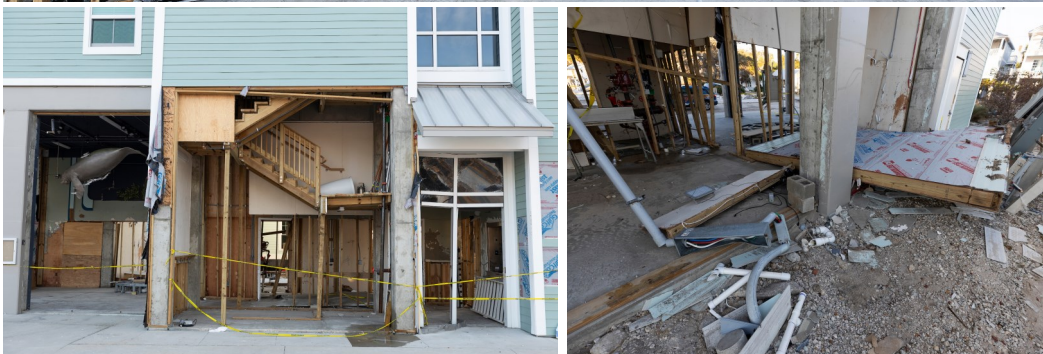
Damage from Hurricane Helene to the UF/IFAS Nature Coast Biological Station.
